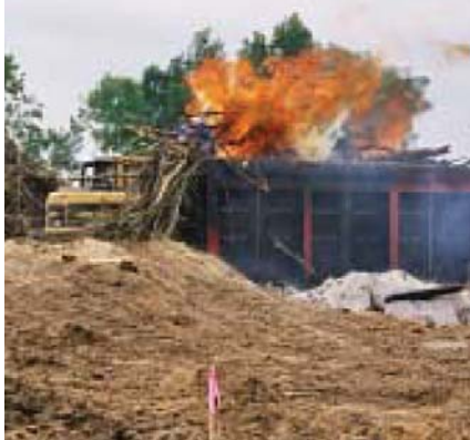
Figure 5: Incinerator box for eradication of nuisance vegetation (ATM, 2004b).
