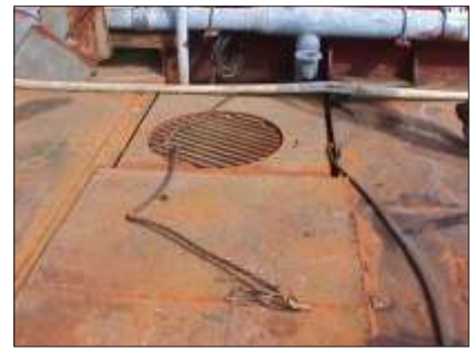
Floor drains and screens
