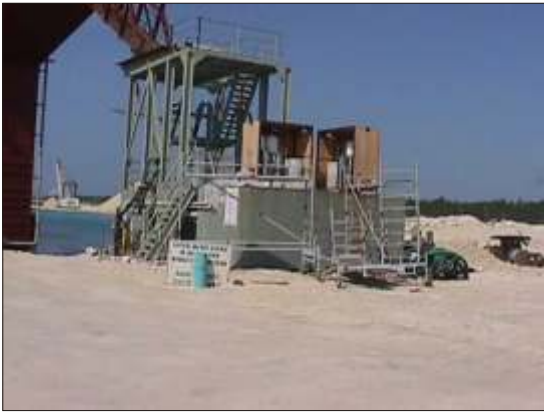
Cascade filtration system
