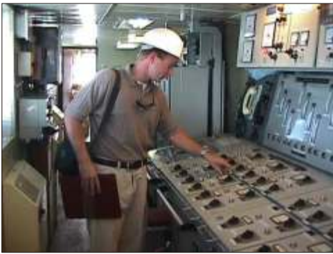
ATM's James Craven inspects dry dock control systems
